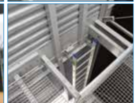
Internal service platforms*
