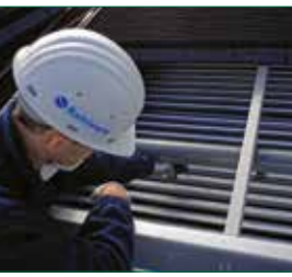
Full access to spray distribution system
